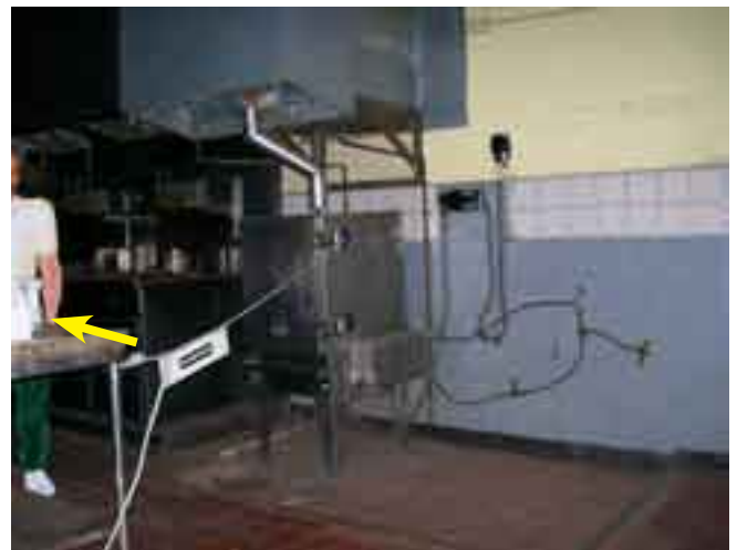
The original positioning of the PIR sensor in the kitchen.
