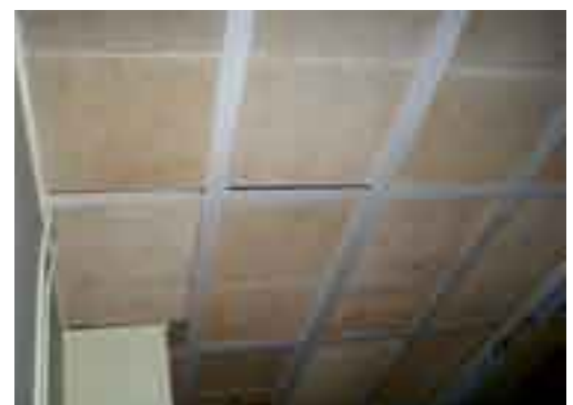
The open “false roof” of the kitchen. The actual raised ceiling (and floor of the 2nd level) is considerably higher.
