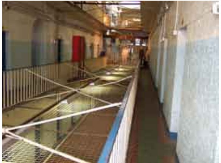
Level 2 West showing the bent cross beam (centre) where a falling inmate collided.
