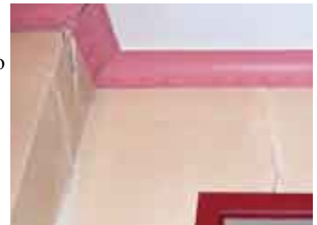
Evidence of structural movement in areas of the building.
