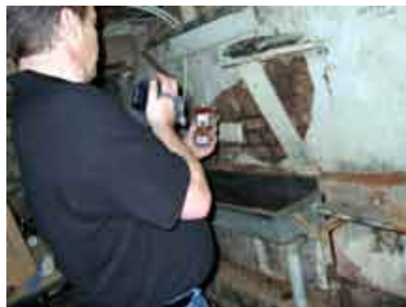
The cellar, with a team member examining the area just after the "blast of air" was experienced.
